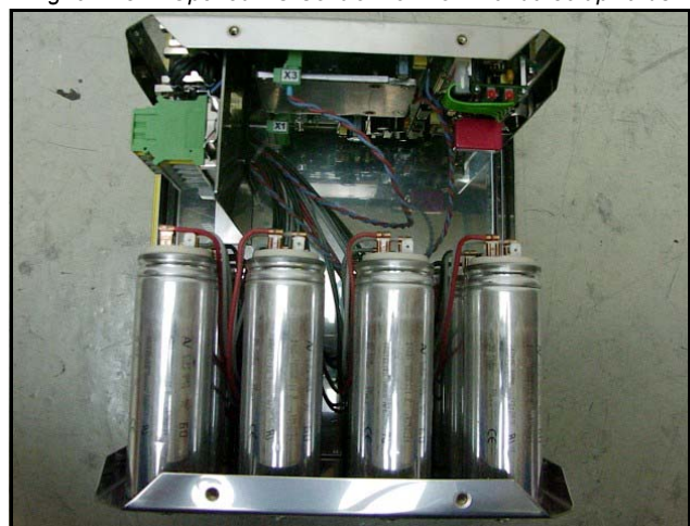
Fig. 6.11.3-2: Opened AC Control Box from Panda 30 upwards
