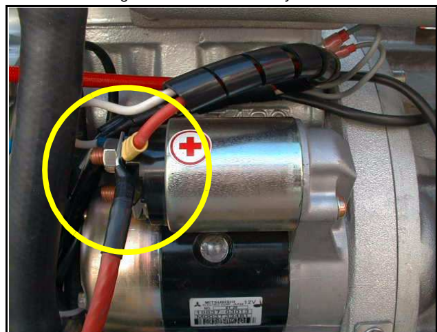
Fig. 5.9.1-1: Positive Battery Cable
