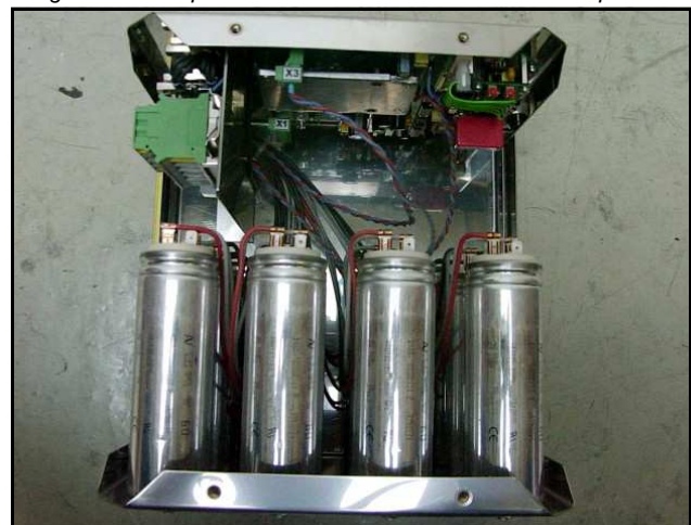
Fig. 5.10.3-2: Opened AC Control Box from Panda 30 upwards
