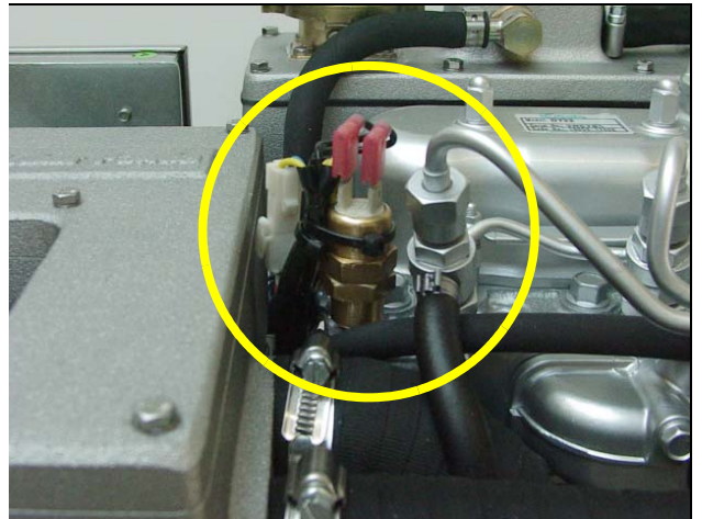
Fig. 4.3.6-1: Thermo-switch at cylinder head
